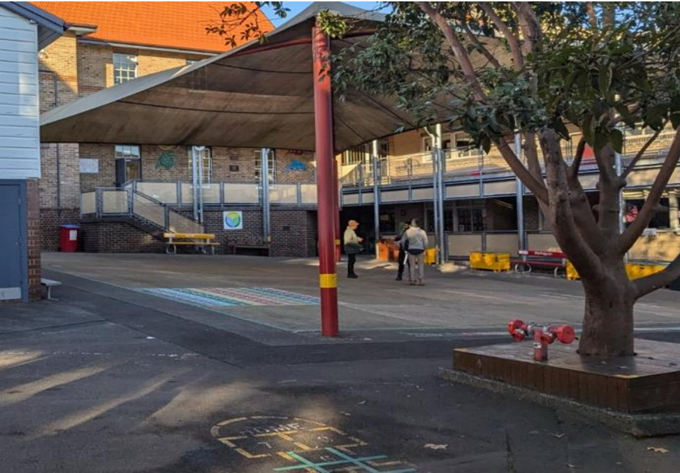
Existing External Fire hydrant (west of Block F):
